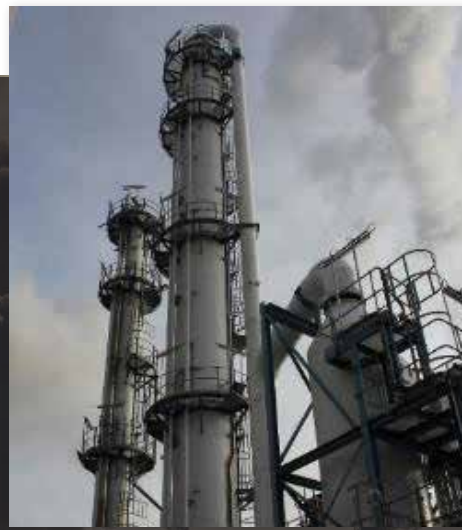
Ferrybridge Carbon Capture Pilot Plant based on Delta Technology, UK
