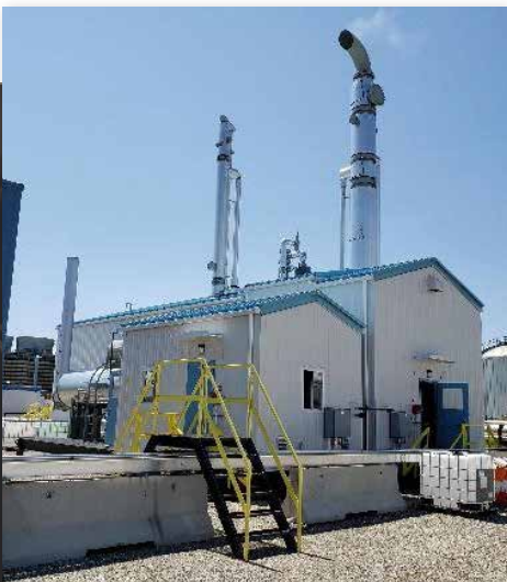
ACCTC Carbon Capture Unit in Alberta, Canada (2020)
