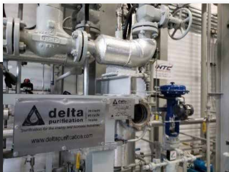
Delta Reclaimer® at ACCTC Site, Calgary, Alberta, Canada
